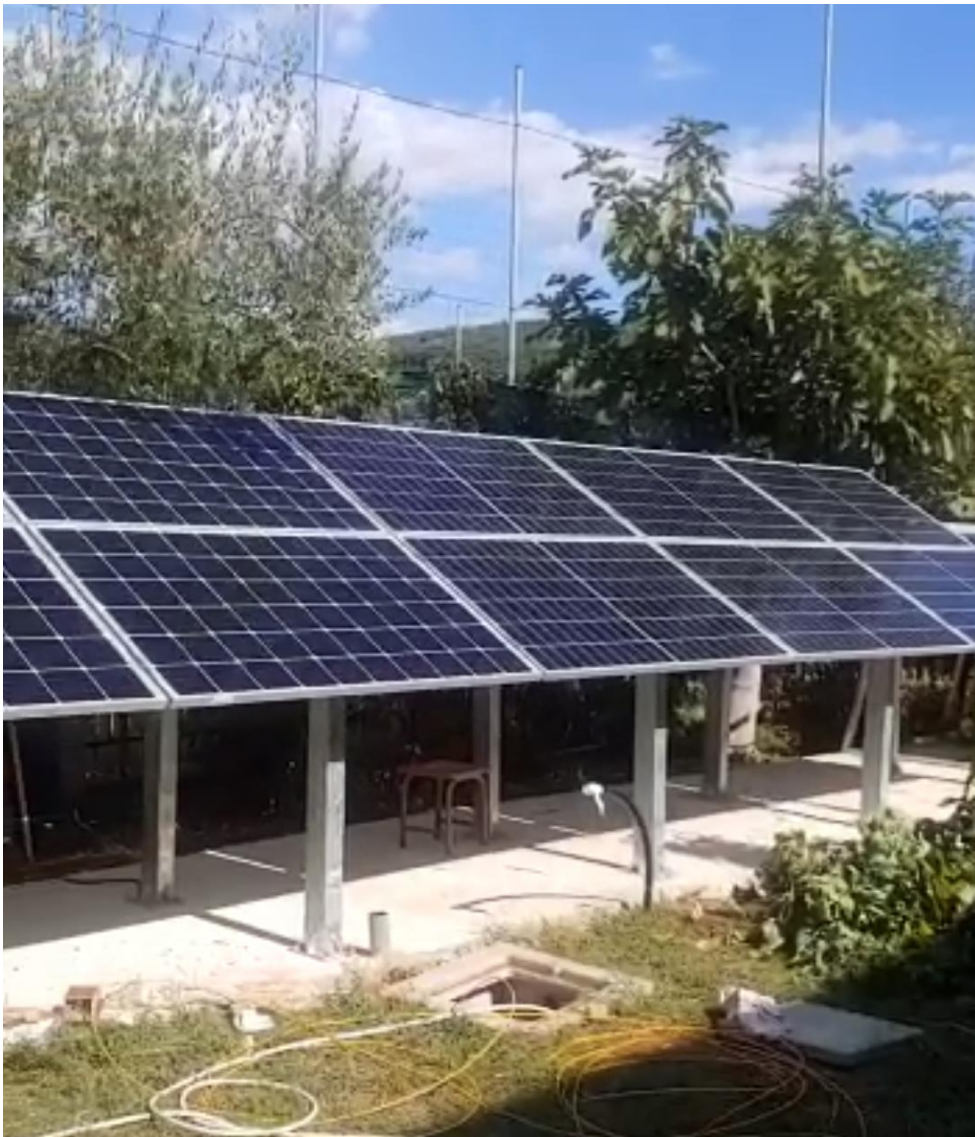
DS700 with solar installation 4,2kW and 10kWh of battery storage
